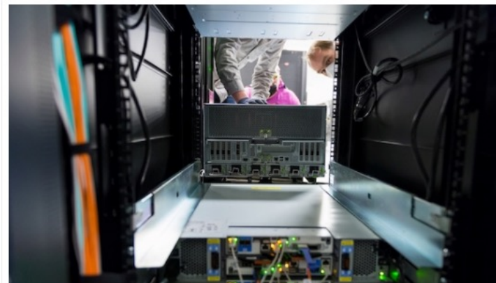
ALCF staff members augment Theta with the installation of NVIDIA DGX A100 nodes. (Image: Argonne National Laboratory)
